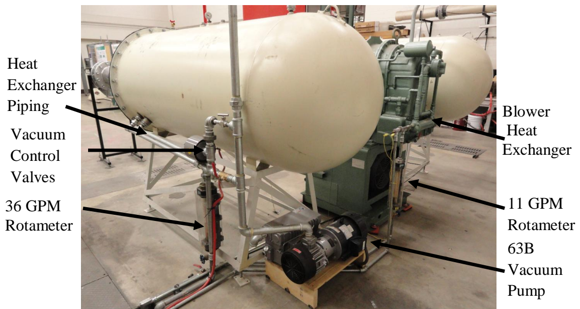
Figure 13. Heat exchanger and vacuum pump systems used during wind tunnel operation.
